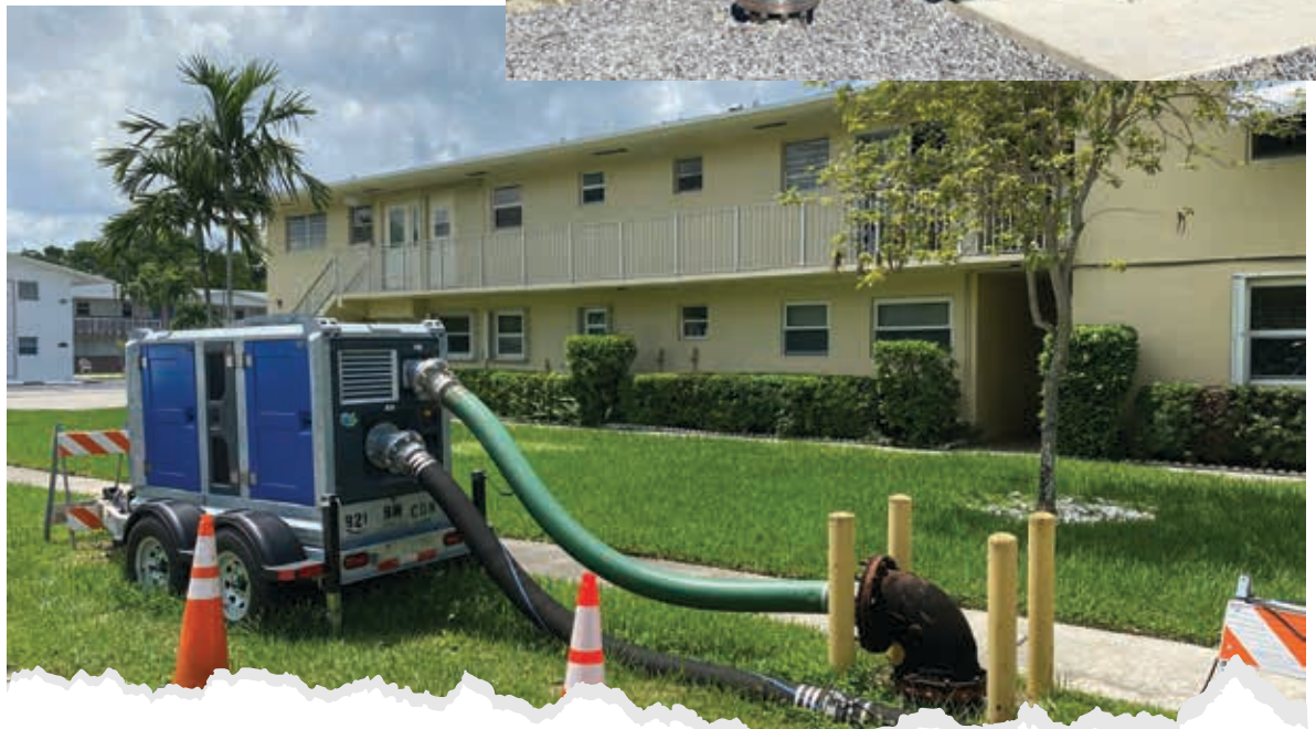
Pump: Mobile Pump on FSA23-EQU21.1
