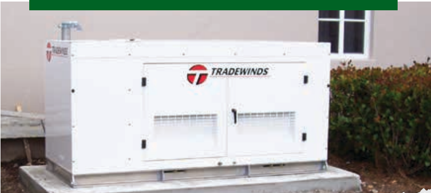
Generator: 125kW Stationary on FSA23-EQU21.1
