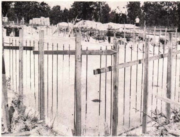
BOYS RANCH SWIMMING POOL —Work is progressing on the olympic size swimming pool which is being built at the Florida Sheriffs Boys Ranch with funds donated by Pinellas County citizens. When Sheriff Don Genung saw the need for a pool some eight or ten months ago, he started the Pinellas County Athletic and Pool Fund which now totals over $25,000. (Sheriff's Star staff photo.)
